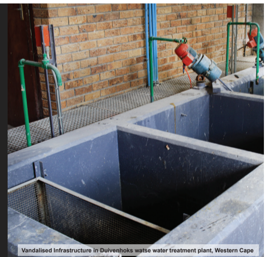
Vandalised Infrastructure in Duivenhoks watse water treatment plant, Western Cape
